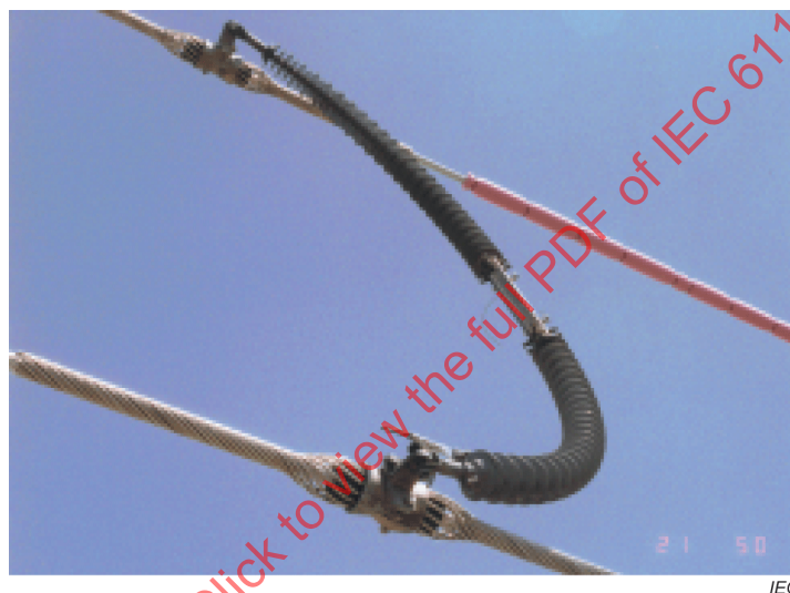
Figure C.2 – Buckling of composite insulator in a phase-to-phase configuration
