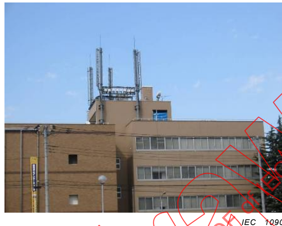
Figure P.5 – Roof-top case study with large antennas and no direct access
