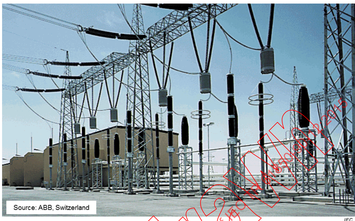
Figure 27 – HV PLC coupling with suspended line traps
