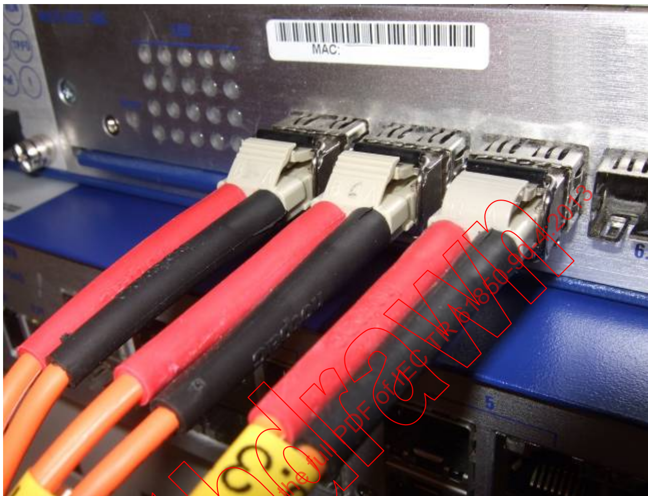
Figure 17 – Switch with optical fibres (LC connectors)
