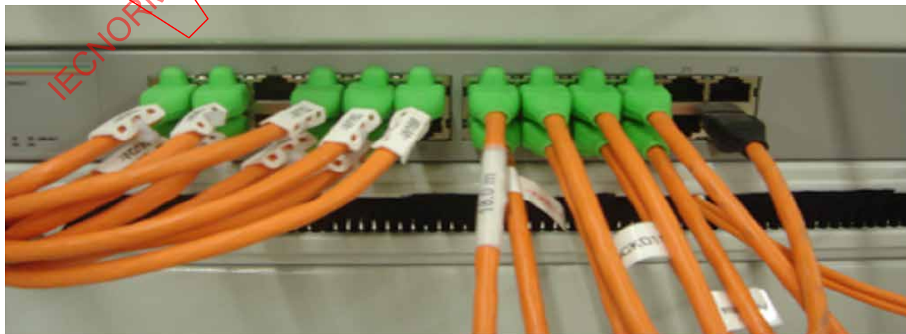
Figure 14 – Switch with copper (RJ45) ports)
