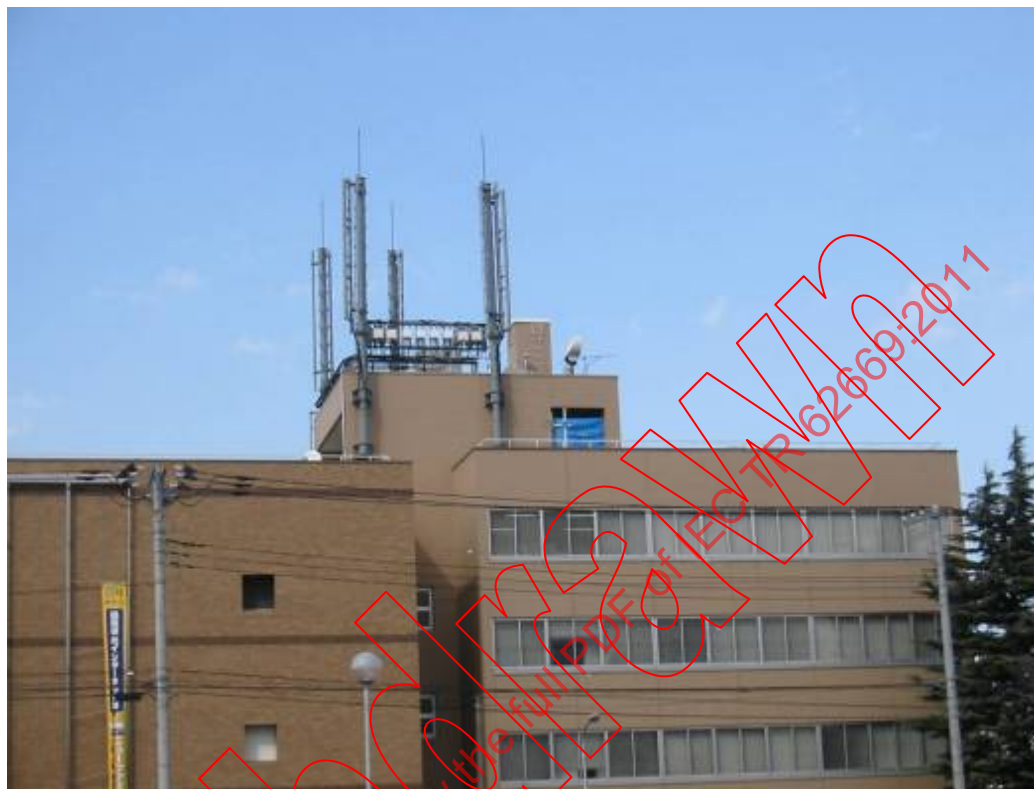
Figure 2.3 Photograph of base station on building roof-top
