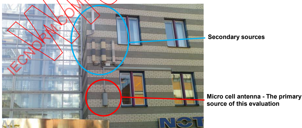
Figure 2.2 Photograph of micro cell antenna
