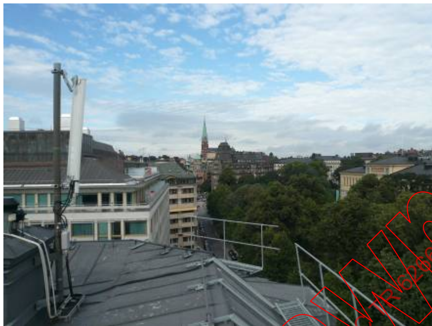
Figure 1: Photograph showing the base station antenna subject to assessment.
