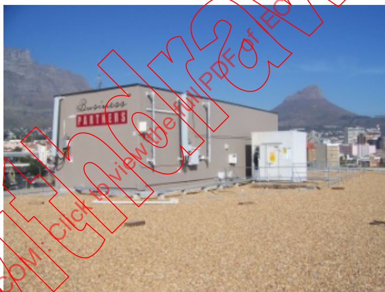
Figure 2.2 Photograph of macro cell on building roof-top antenna
