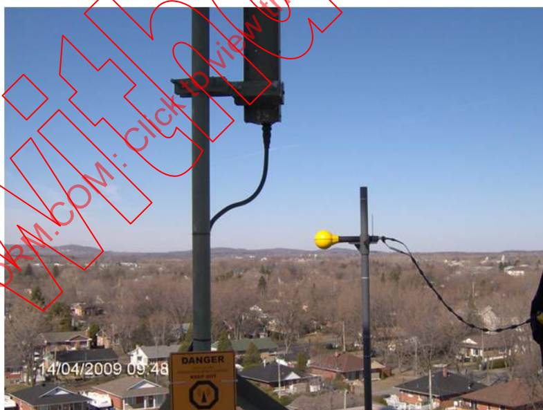
Figure 4: Location J in front of the satellite broadcasting repeater
