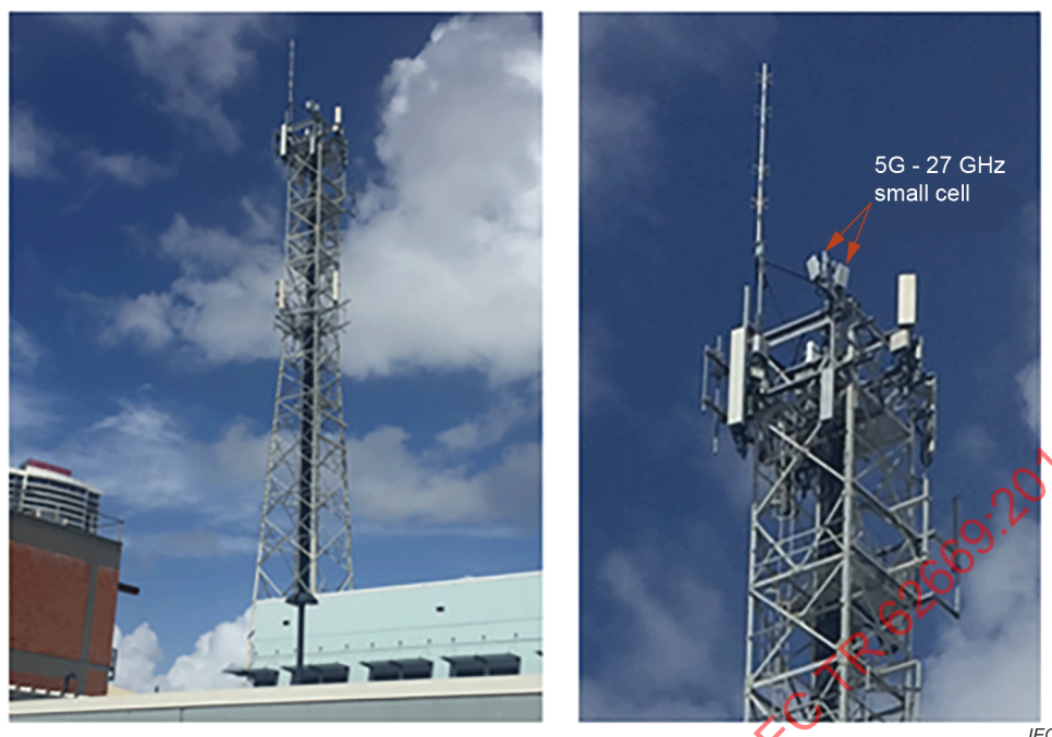
Figure 30 – Outdoor site with 5G small cell product at millimetre-wave frequency installed on a 44 m radio tower
