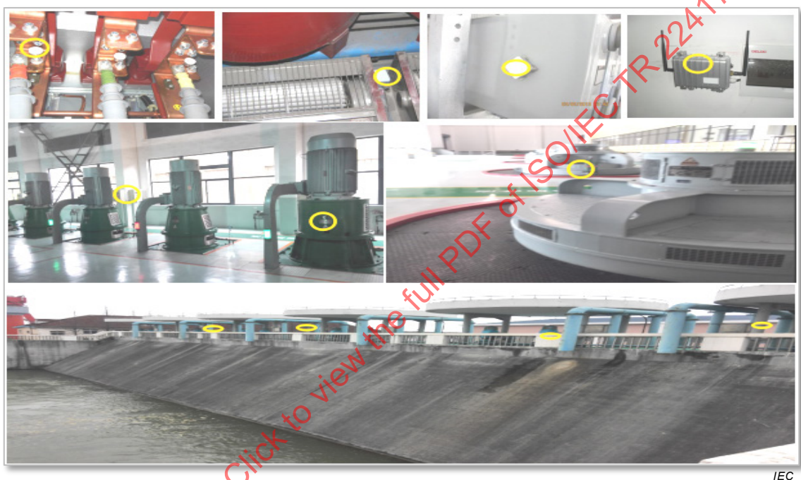
Figure 41 – Monitoring and Control System in Water Plant project in Shanghai
