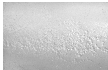
Figure B.4 — Line corrosion
