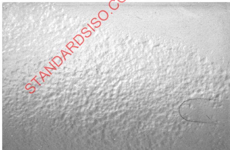
Figure B.3 — General corrosion
