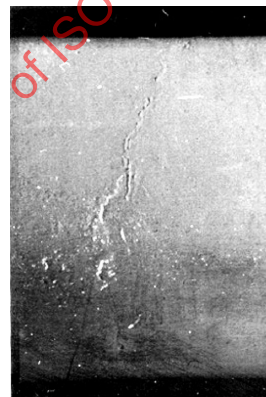
Figure B.2 — Crack
