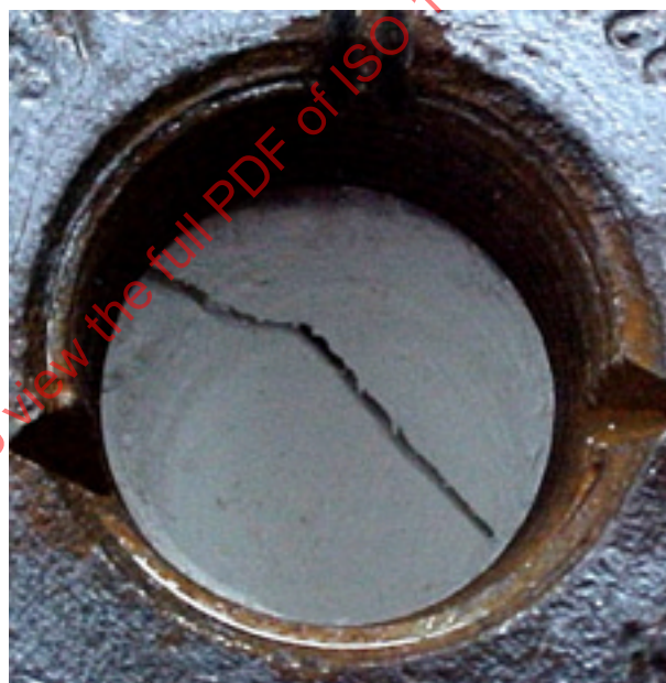
b) Crack with visible sidewalls
