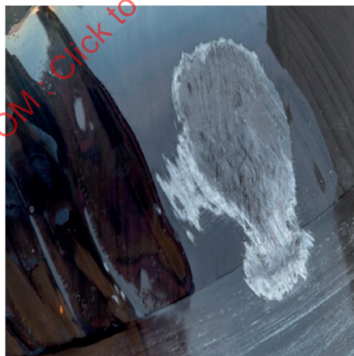
c) Examples of Level 3 abrasion damage
