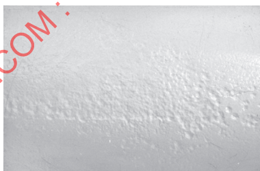
Figure B.4 — Chain pitting or line corrosion
