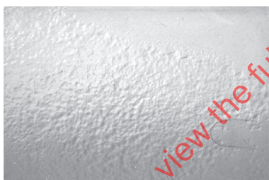
Figure B.3 — General corrosion
