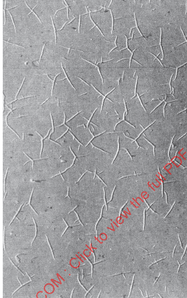
Figure 8 — Crow's foot cracking
