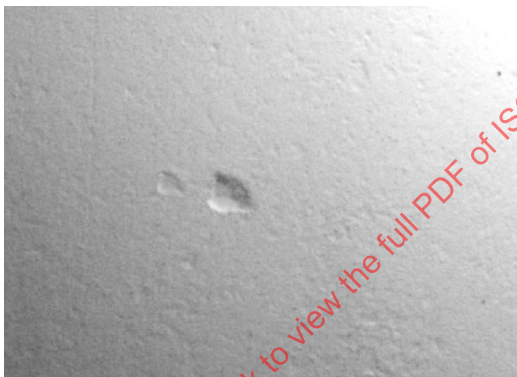
Figure B.5 — Isolated pits
