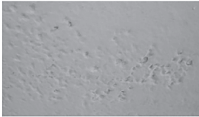
Figure A.14 — Pitting
