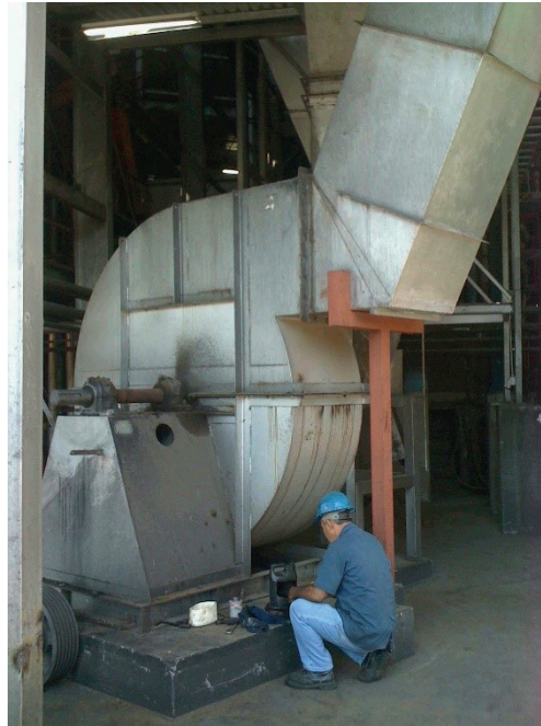
Figure 39 — Poor outlet elbow installation
