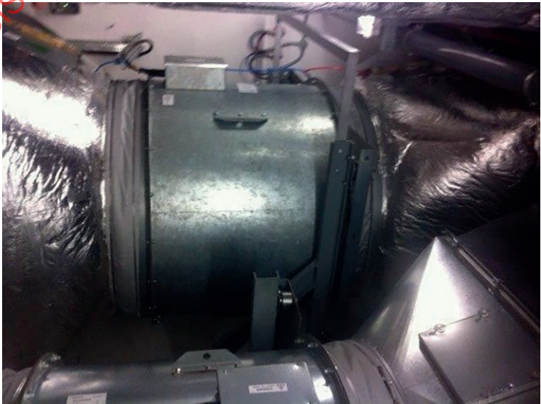
Figure 41 — Example of poor inlet/outlet conditions
