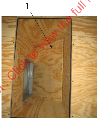
Figure 21 — Return fan inlet cabinet with perpendicular right-side wall at 0,25D from the impeller
