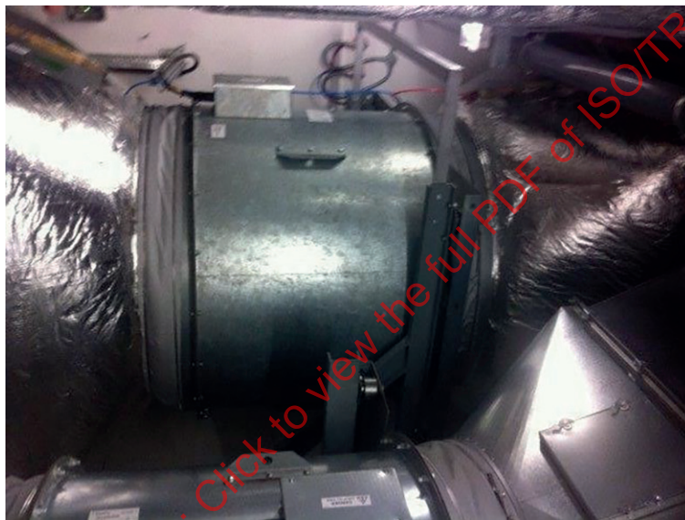
Figure 41 — Example of poor inlet/outlet conditions
