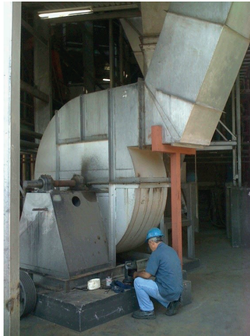
Figure 39 — Poor outlet elbow installation
