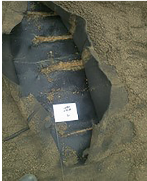
Figure 3 — Barrier damage due to construction traffic
